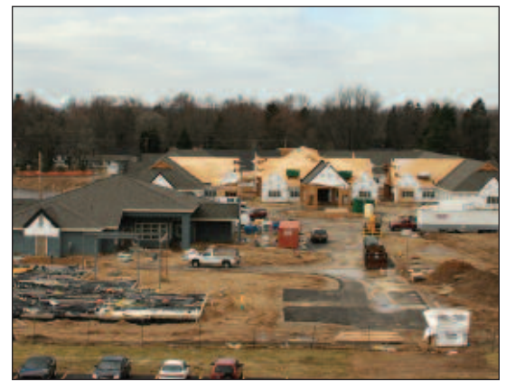
Spring construction continues to shape Borgess Gardens, slated to open late this fall or early winter.
